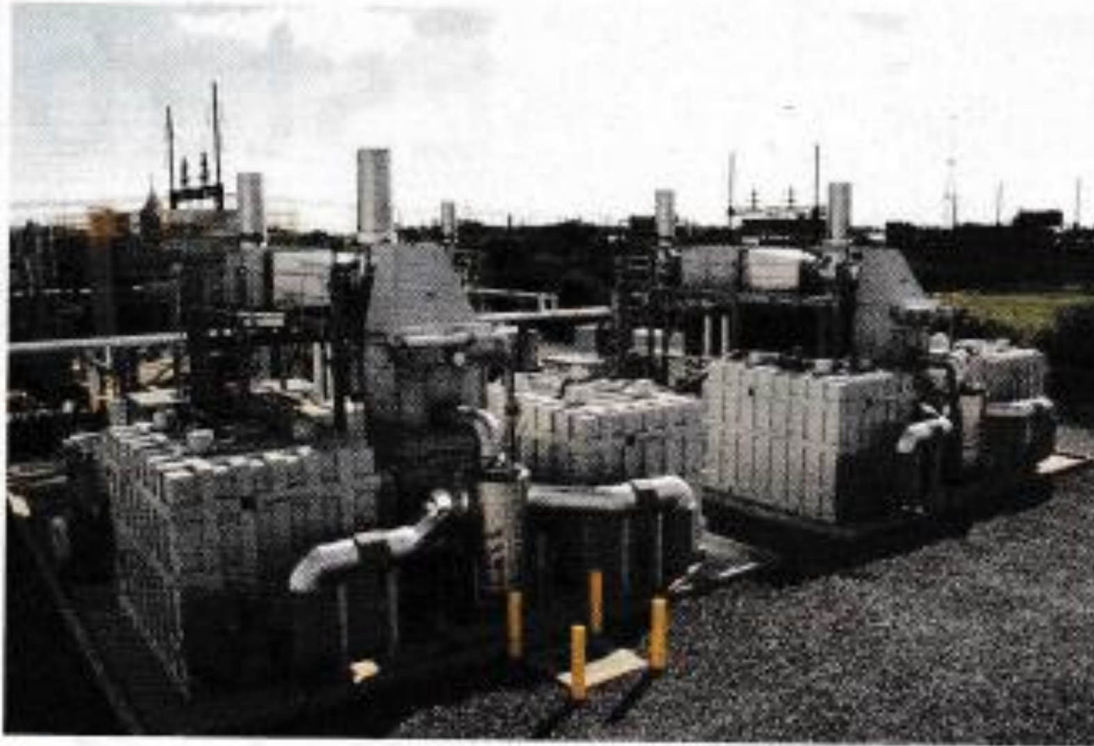
▲ Figure 3. These 15-MW molten carbonate fuel cells (MCFCs) began operation in Bridgeport, CT, in 2013. Photo courtesy of Fuel Cell Energy.
