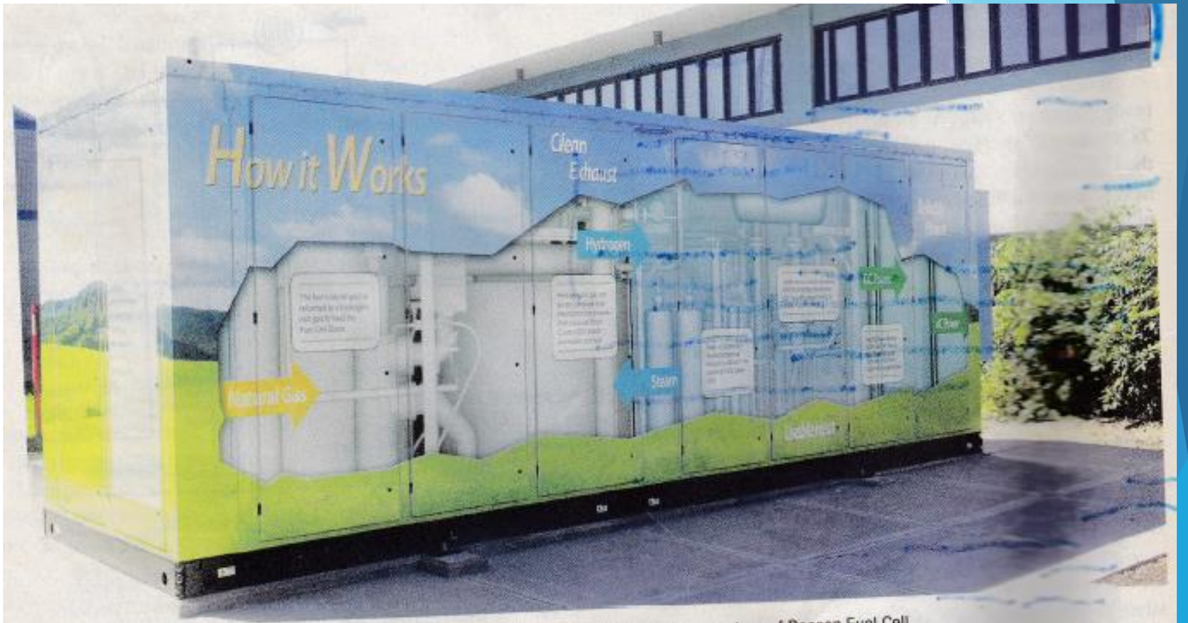
▲ Figure 2. This 400-kW phosphoric acid fuel cell (PAFC) produces hydrogen onsite. Photo courtesy of Doosan Fuel Cell.
